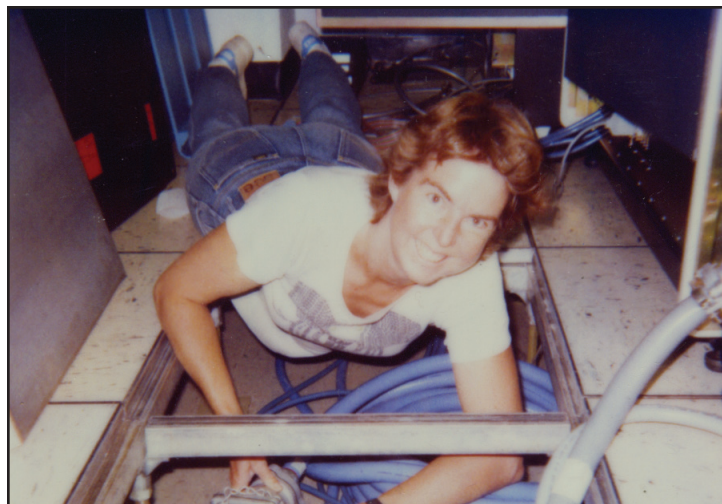
Chela Kunasz laying cables in 1988 for the VAX8600 computer under the subfloor of JILA's new computer room in the basement of the new S-wing laboratory building. Credit: JILA
