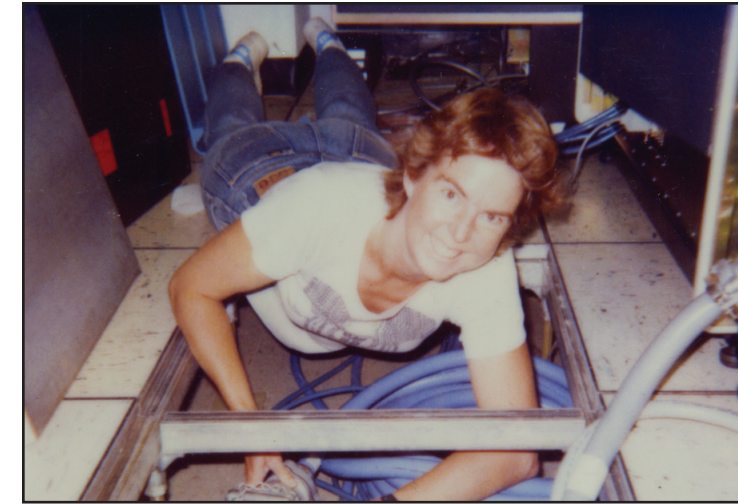
Chela Kunasz laying cables in 1988 for the VAX8600 computer under the subfloor of JILA's new computer room in the basement of the new S-wing laboratory building. Credit: JILA
